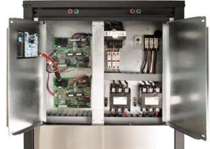
Advanced digital controls with Remote Service Sentinel and compressor "run" and "fault" LED. Optional Enhanced controls (DXM) & DDC Controllers
